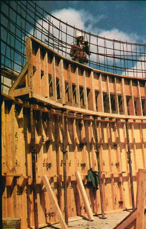
The floor slab of a clarifier and the forming of its walls at Balmertown, Ontario.
