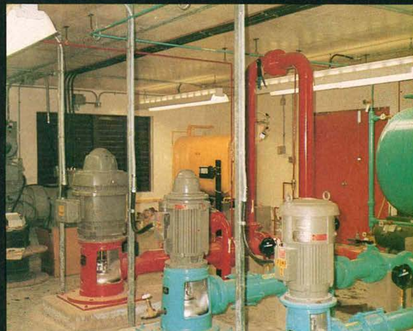
The mechanical system of a water treatment plant at Bloodvein.
